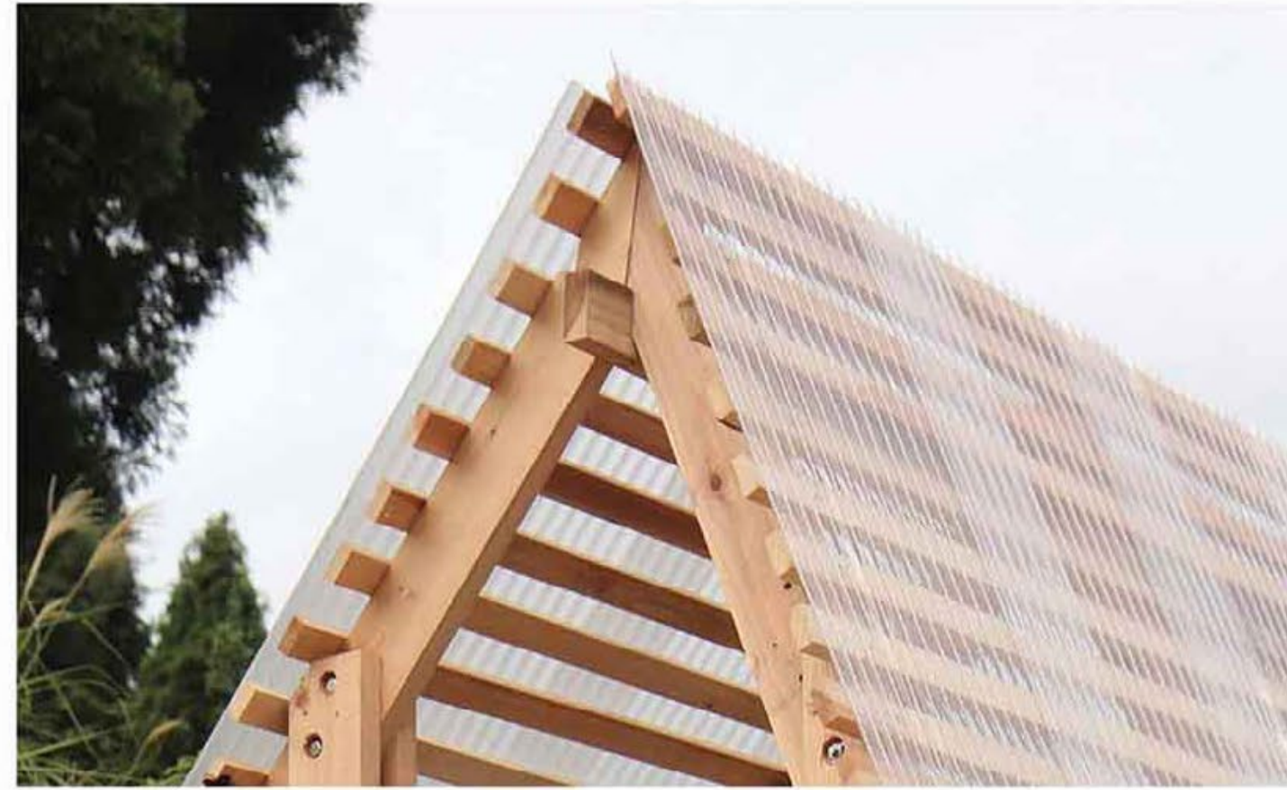
Exposed timber truss roof with a polycarbonate covering for diffused light filtration
