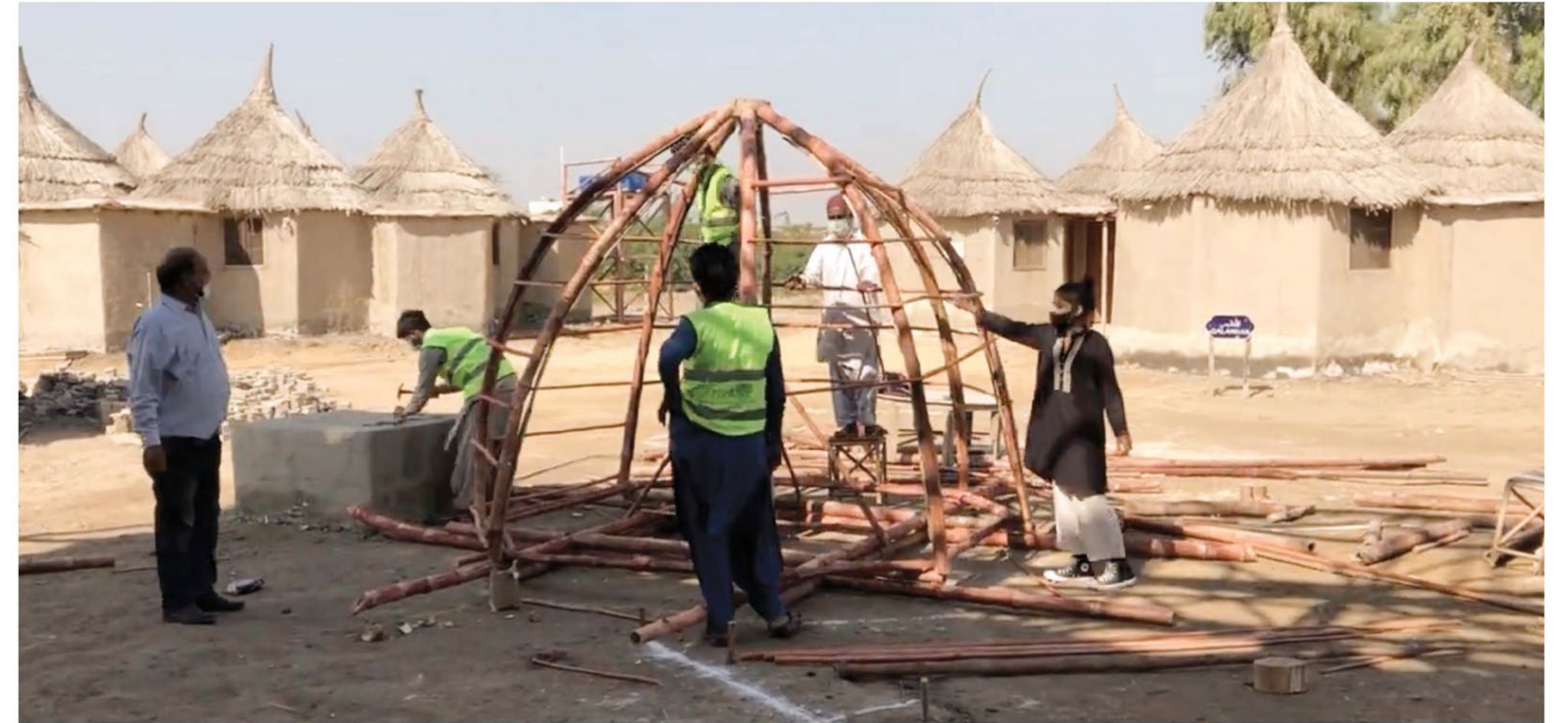
Bamboo pod typology constructed at Yasmeen Lari's 'Zero Carbon Centre Design Lab in Makli, Pakistan
