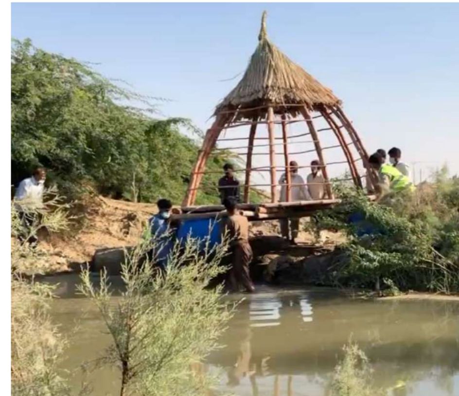
Bamboo pod covered with that roof to provide shade before submerging into canal
