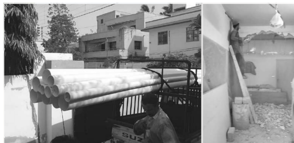
The primary work was the internal fit-out, involving reinstalling plumbing and electrical systems throughout the house, adjusted a revised spatial layouts
