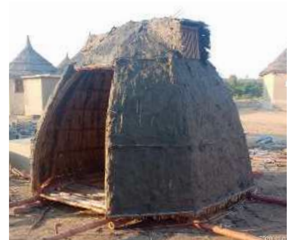
Bamboo Pod clad with thin layer of earth-lime plaster to provide shelter
