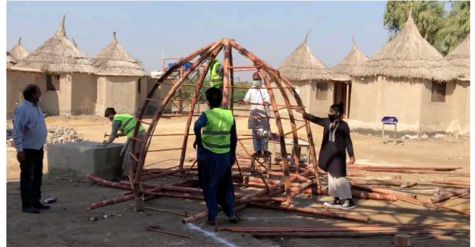
Bamboo pod typology constructed at Yasmeen Lari's Zero Carbon Centre in Makli
